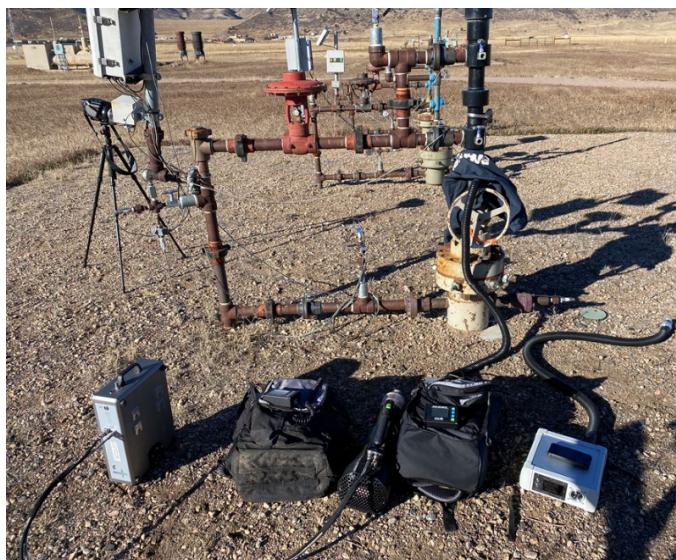
Figure 30: HFS units at METEC. Left to right: Sensors, Inc. (gas sensor module, handheld unit attached by cord), Bacharach HI FLOW, Hetek Flow Sampler, and the AddGlobe GFM.
